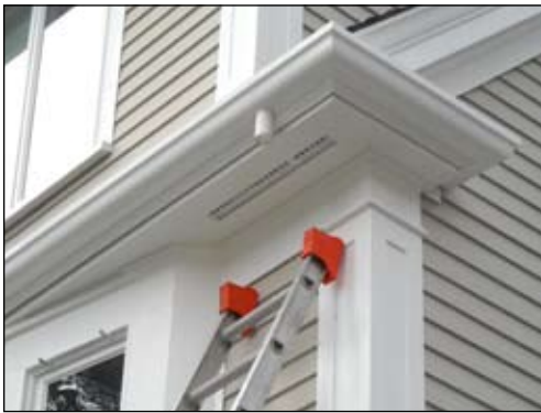
A recent installation of Boston Proper™ fiberglass gutter by Architectural Composites of New England on an historic Duxbury, Massachusetts home, including a newly constructed addition.
